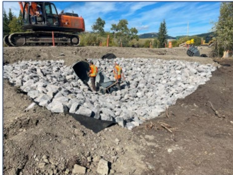
September 23, 2024 Rip rap placement is in progress at the upstream end and the substrate is placed within the culvert.
